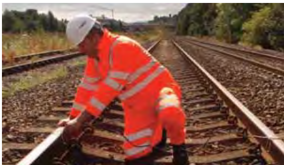
Using a track-circuit operating clip
